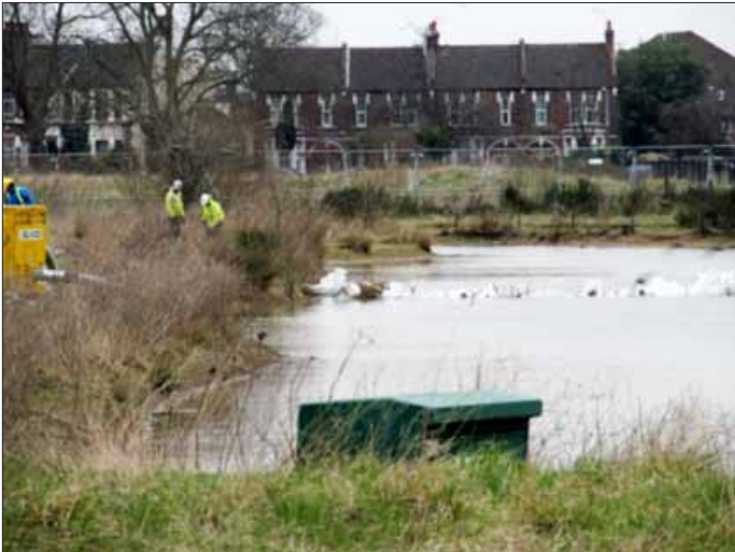
The dam, or bund, going across the narrowest part of the pond, 3rd April 2013
